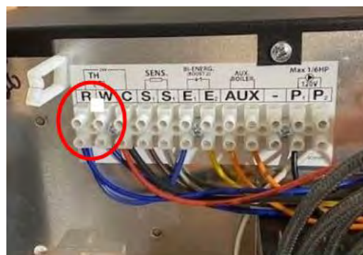
Back Up Terminals on Boiler
