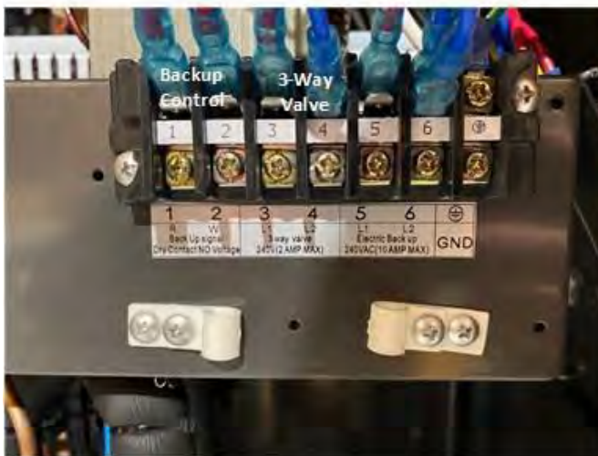
Remove front panel to access accessory terminal block
