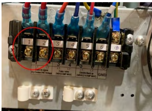
Back Up Terminal on Heat Pump
